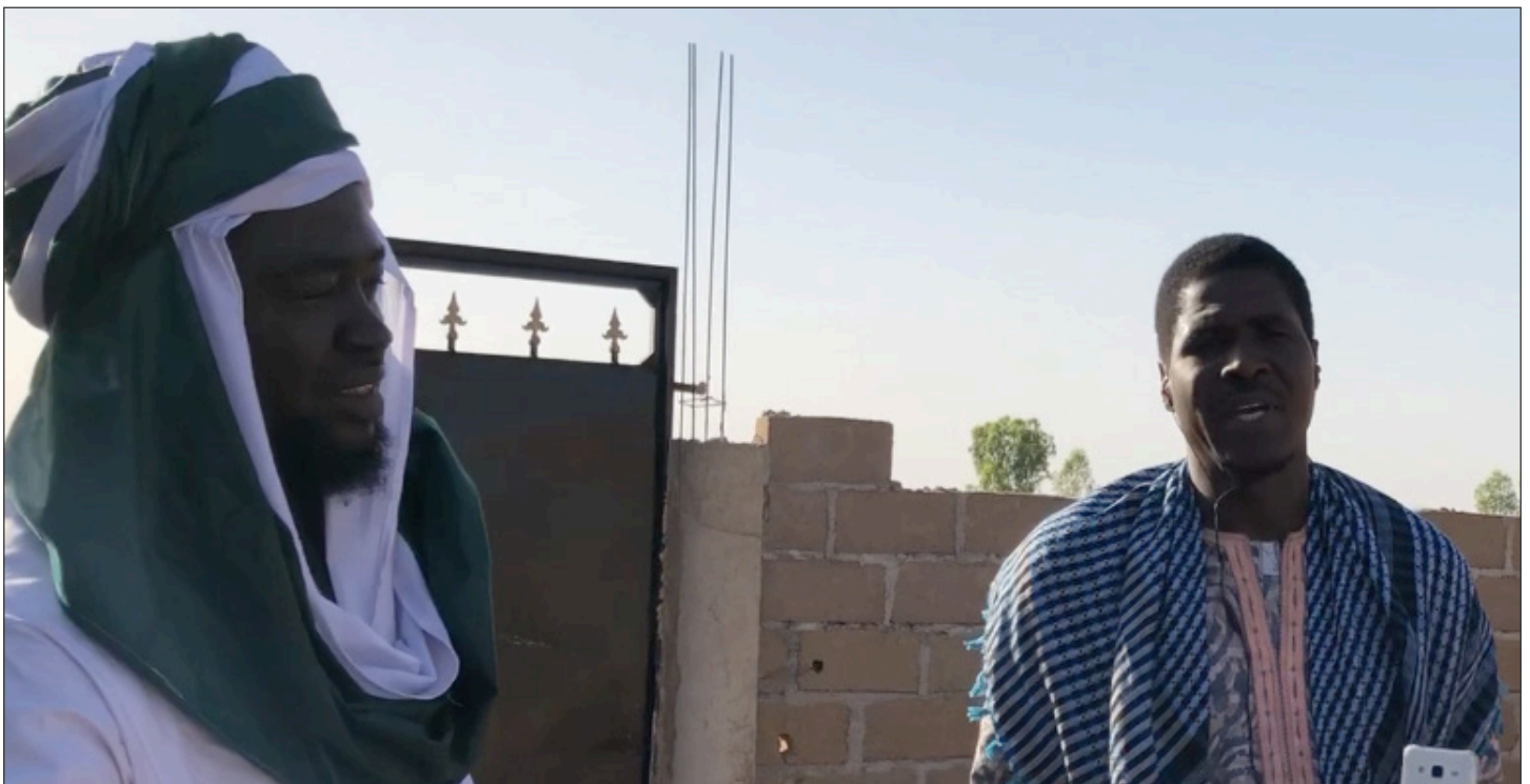
Video clip of Sufi Cheick Bilal and Sufi Cheick Saïdo at the Holy Quran School construction site
